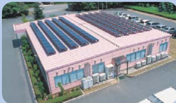
Solar power generating system installed on factory roof
